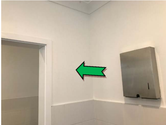
Photo 7. Ladies toilet lobby, south end, west elevation, wall – non asbestos-containing fibre cement sheeting.
