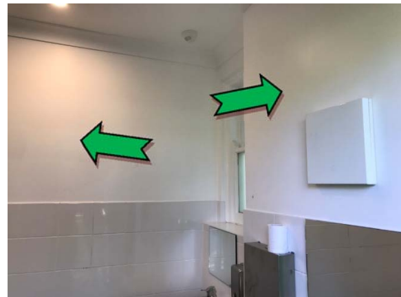
Photo 4. Interior, disabled toilets, north and west wall – non asbestos-containing fibre cement sheeting.
