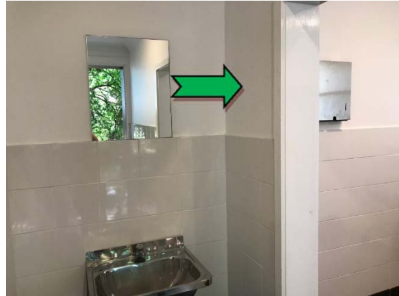
Photo 8. Ladies toilet lobby, south end, east elevation, wall – non asbestos-containing fibre cement sheeting.
