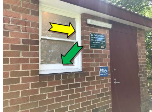
Photo 2. Exterior, throughout, window frames – non asbestos-containing window caulking and suspected lead-containing white upper paint systems.
