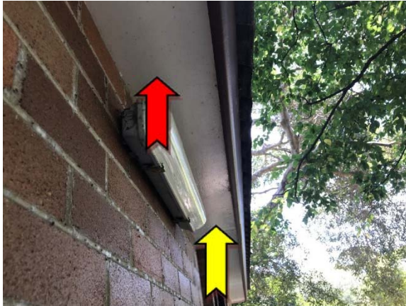
Photo 1. Exterior, throughout, eaves – asbestos-containing fibre cement sheeting and suspected lead-containing white upper paint systems.
