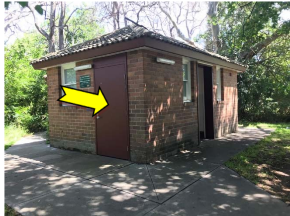
Photo 10. Exterior, throughout, door – suspected lead-containing red upper paint systems.
