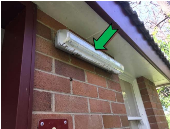
Photo 9. Exterior, throughout, single tubed fluorescent light fittings – suspected non PCB-containing capacitors.
