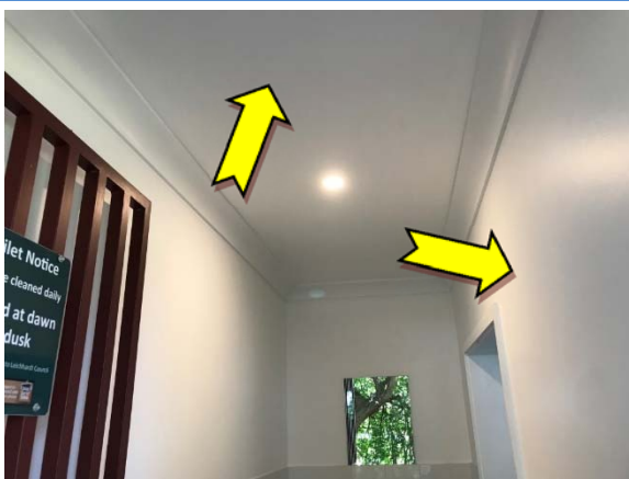
Photo 11. Interior, throughout, walls and ceilings – suspected lead-containing white upper coloured paint systems.
